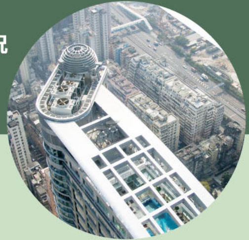
朗豪酒店的蒸發式冷卻塔 Evaporative cooling towers at Langham Hotel
